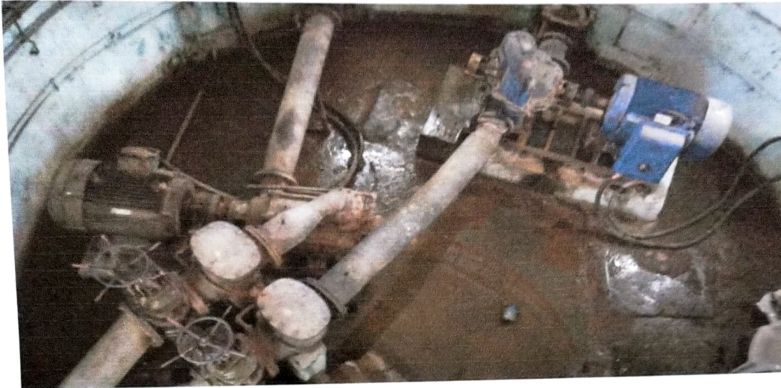
3. The pumps at Water Pump house
