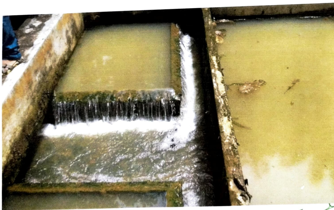
3. Water over flowing from Sedimentation tank at Site
