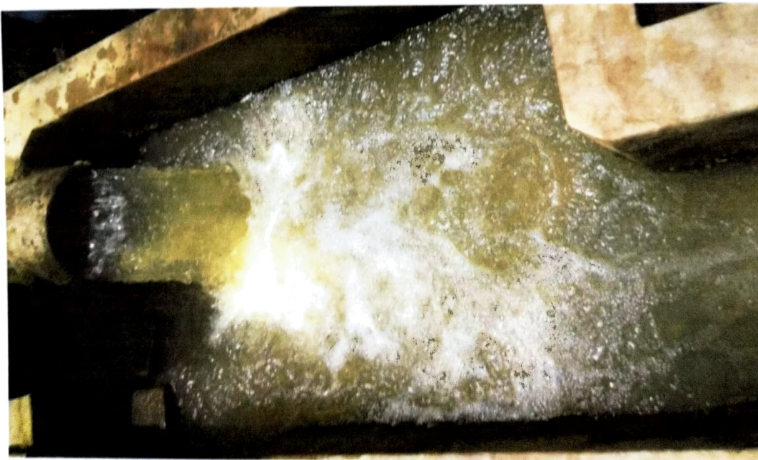
1. Water inlet into the Tank
